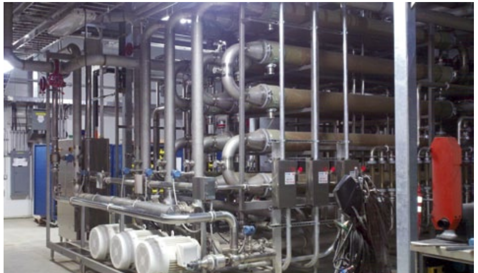
Wastewater treatment system with Berghof external AnMBR technology
